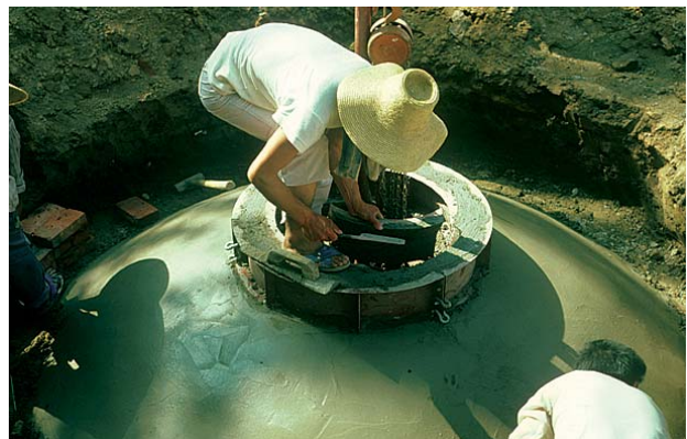
Small-Intermediate Scale Digester
